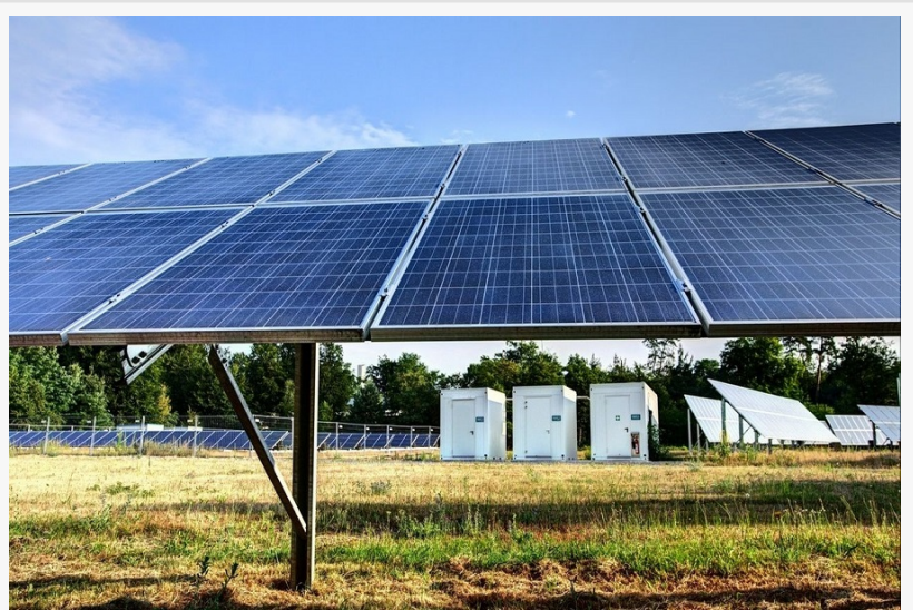
Renewables Battery Energy Storage Market
