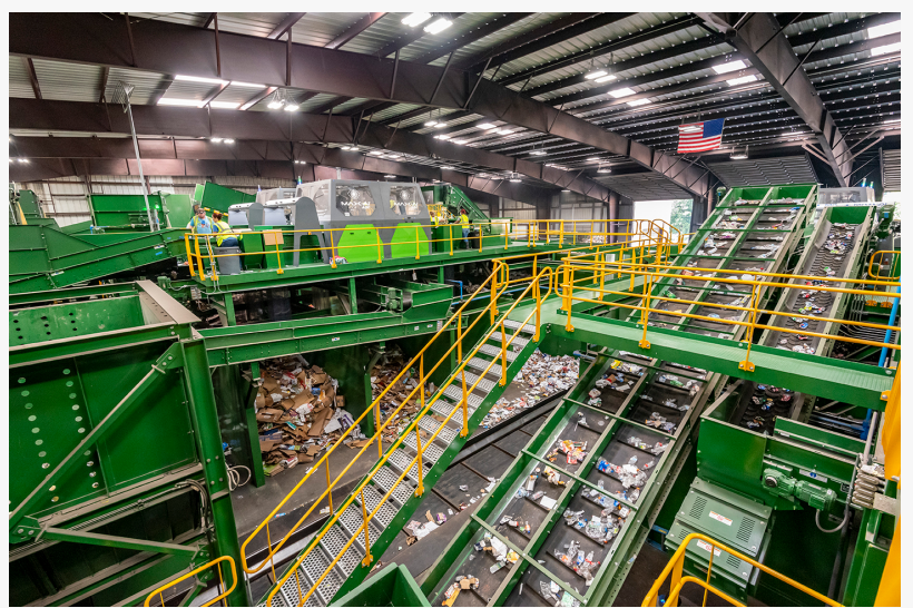
Tulsa's Murph 2.0 Recycling Facility
