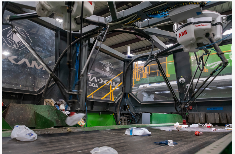
Recycling Facility, Equipped with Recycling AI Robots
