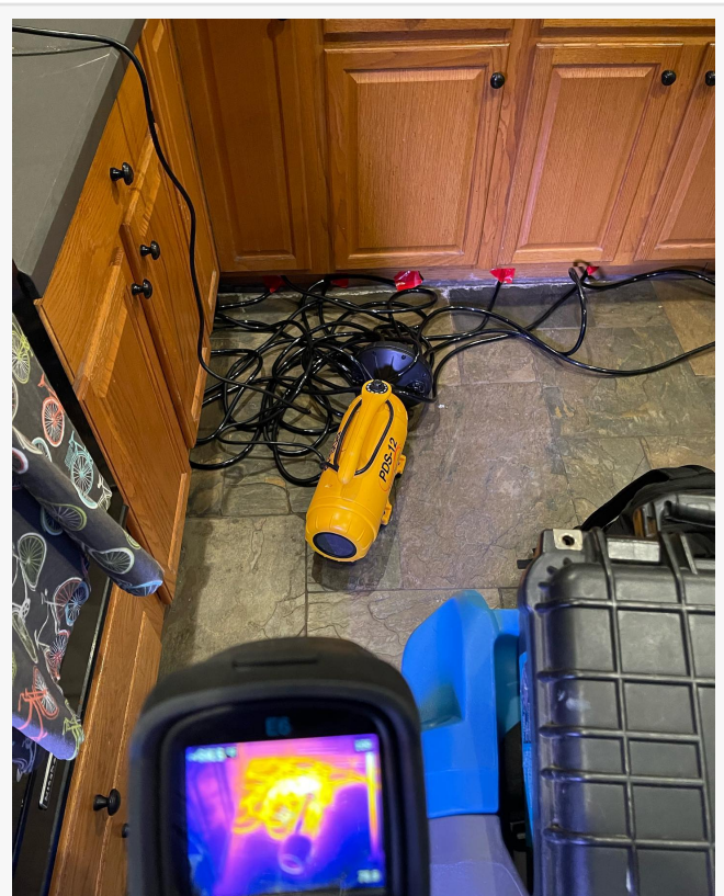
gilbert az water damage clean up
