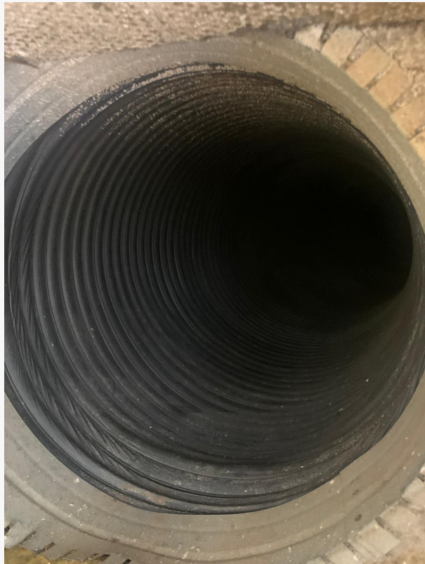
Clean Quality Air Duct Cleaning PSL
