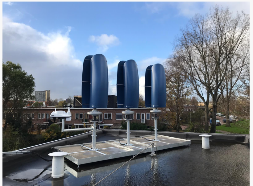
Three installed small size Wind Tulips
