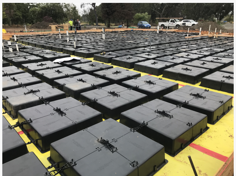
Waffle Boxes on Grade awaiting concrete to be poured for NorthStar Luxury Homes
