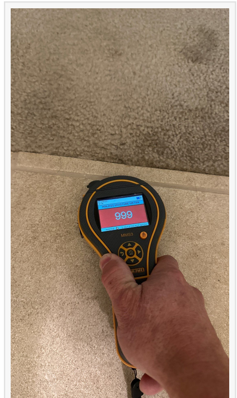
Moisture reading showing that there is water damage.
