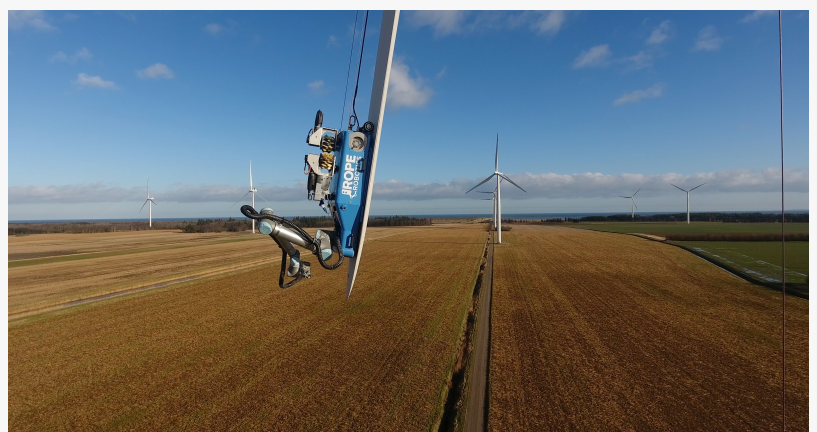
Rope Robotics' robot is the first commercial robot to automatically repair the leading-edge of the blade.
