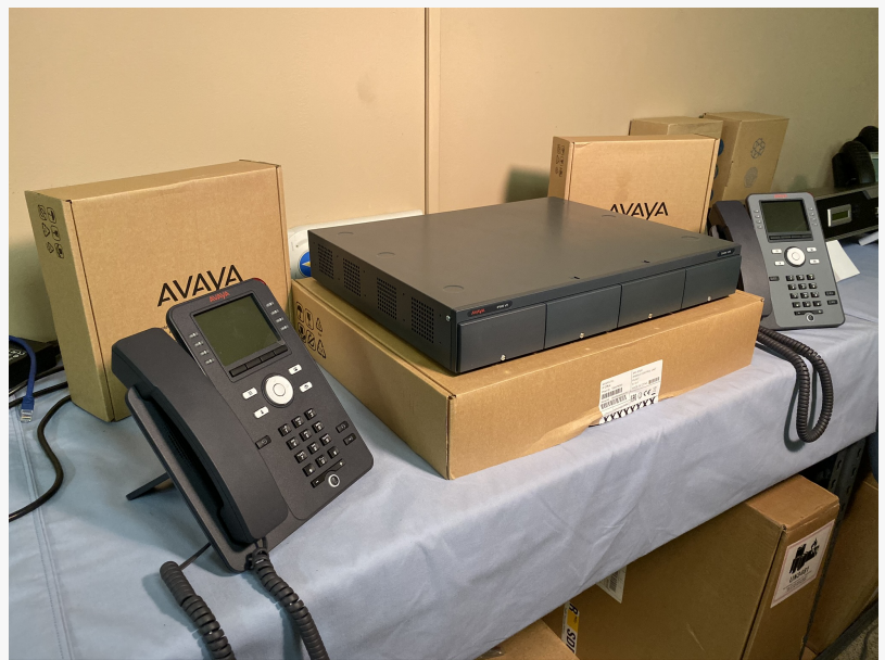
Avaya IP Office stationed in Lanstar Voice & Data, LLC's office - Ready for deployment
