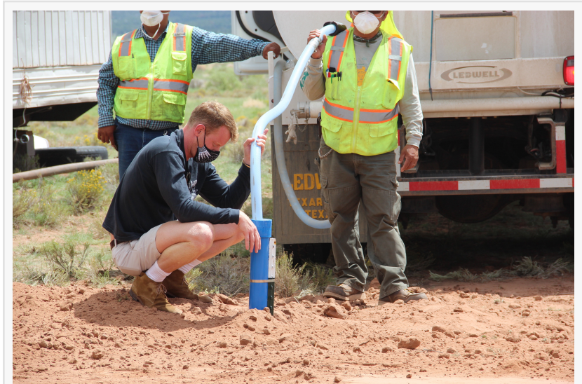
George McGraw, founder and CEO of DigDeep, helps to fill a newly installed Home Water System with fresh, clean water on the Navajo Nation.
