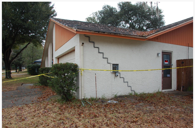
USGS photo of home damaged by sinkhole
