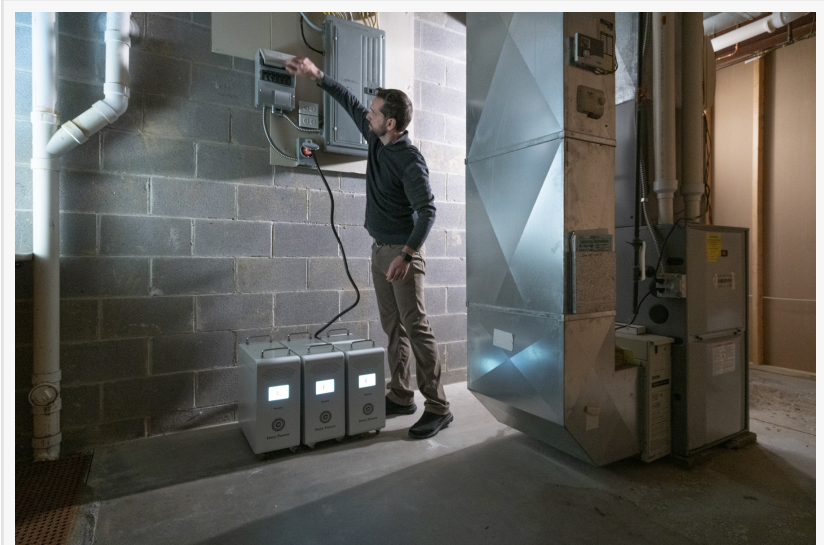
Backup home furnace and appliances
