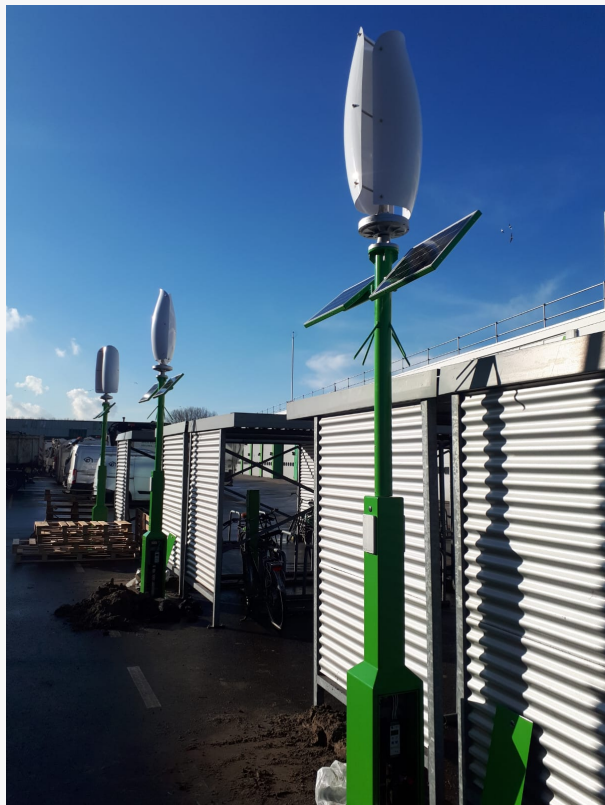
Wind and Solar E-bike Charging Poles
