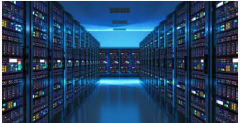
Colocation Data Center Market
