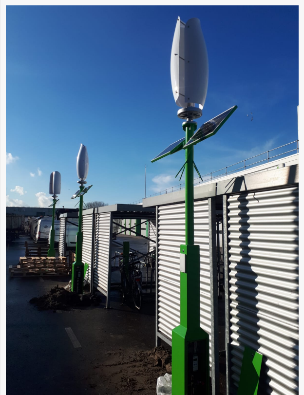
Wind and Solar E-bike Charging Poles
