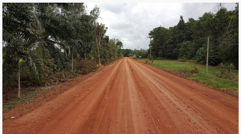
A road in the Pilbara region treated with Titan by RST Solutions remains in excellent condition after rain.
