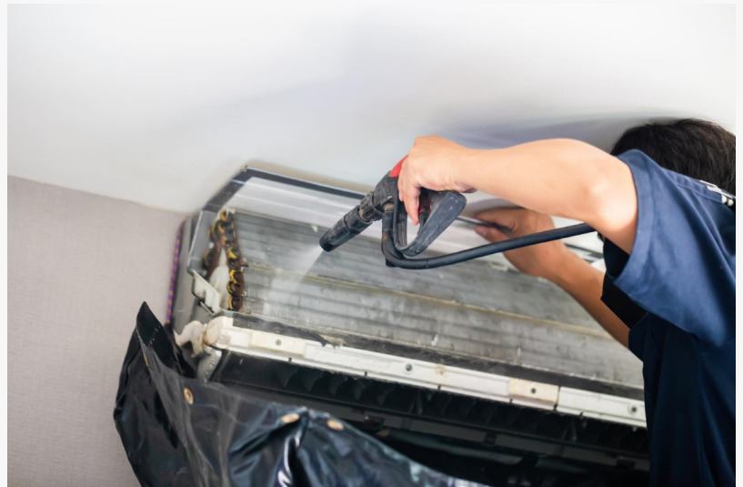
Top-Quality Air Conditioning Services
