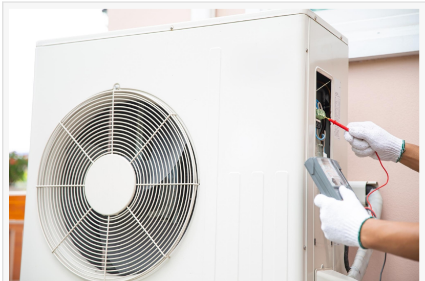
Air Conditioning Services
