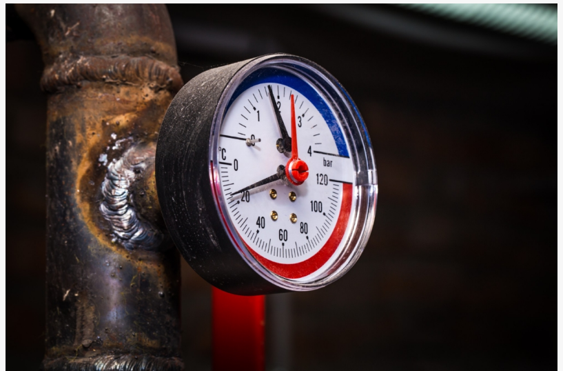
Leak Detection Services in Port St. Lucie
