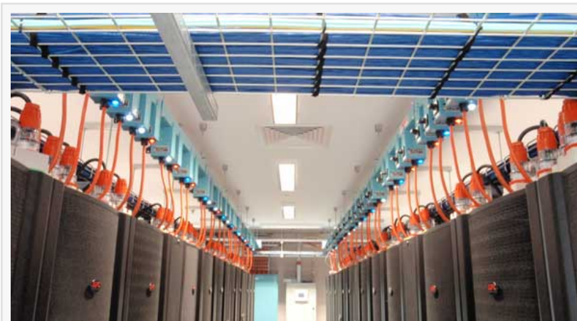
Data Center Busway
