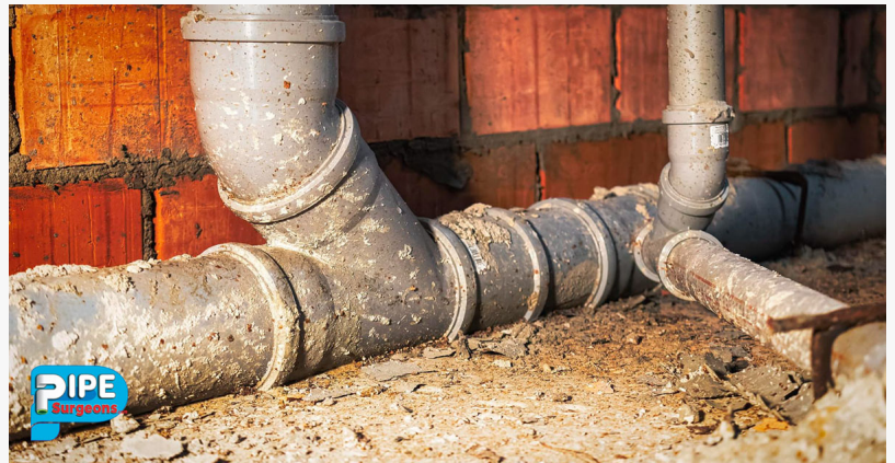
Underground Utility Services in Port Saint Lucie
