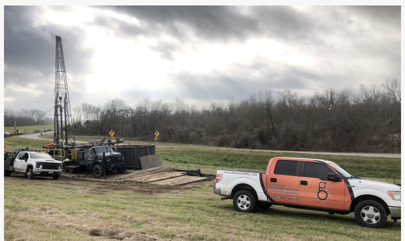
Genesis 360, LLC, works on a contract with the Army Corps of Engineers in New Roads, Louisiana.
