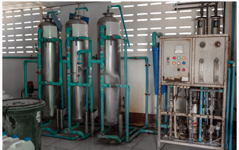
Boiler Water Treatment Chemical Market PMI
