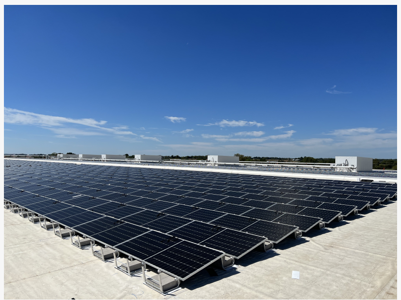
Rooftop Solar Array on ColdPoint Logistics in Edgerton, KS, a NorthPoint Development building
