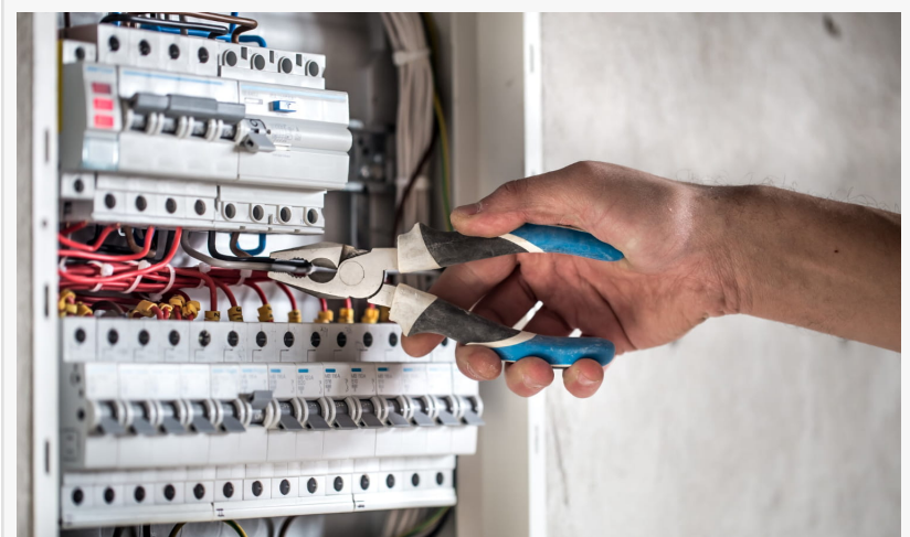
Residential Electrician Services
