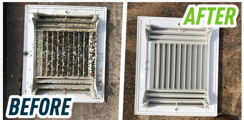
Air Vent Cleaning in Las Vegas
