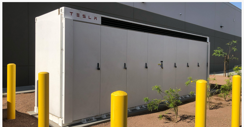
A Tesla Megapack set up as a micro grid provides independence to companies looking to save on energy costs and break from utility dependence.
