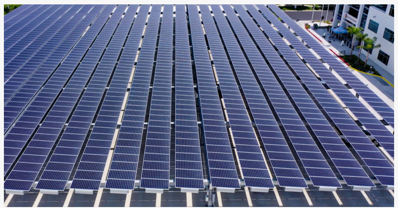
Solar arrays can bring the added benefit of shaded parking when designed as a long span system like this one in San Diego County.
