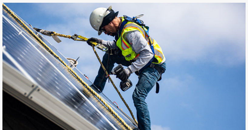
A solar installer working on a steep-pitched roof puts in a solar system during the construction of a new multi-family complex in San Diego County
