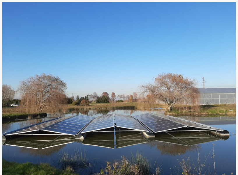
Upsolar Floating FPV plant in Venice, Italy
