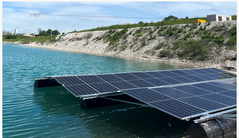
Upsolar Floating FPV plant in Treviso, Italy
