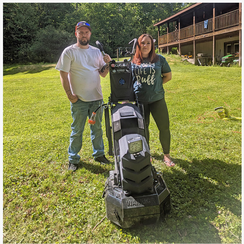
Cody & Ashley Miller pictured with their new Warrior Equipment Black Ops Tomahawk concrete grinder.
