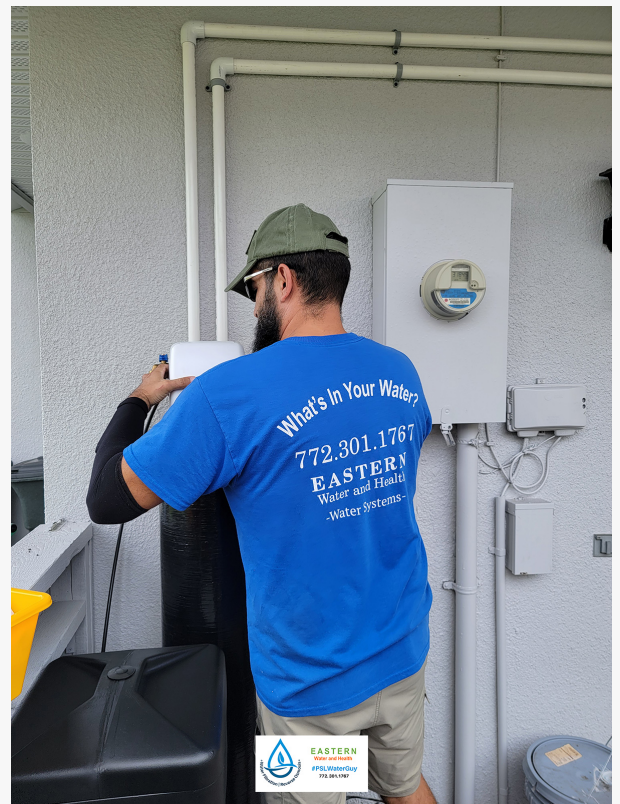
Water Treatment Installation Professionals in PSL
