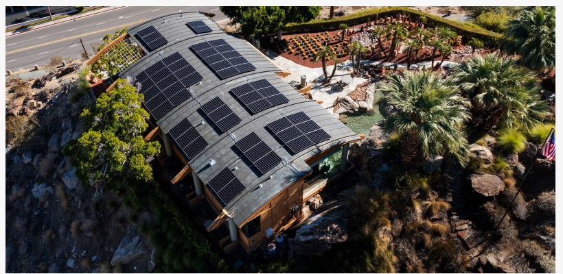
Residential Solar for MMR
