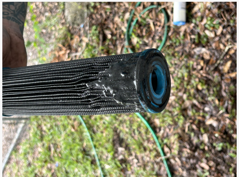
Sediment Filter Needing Replacement in Lakewood Park
