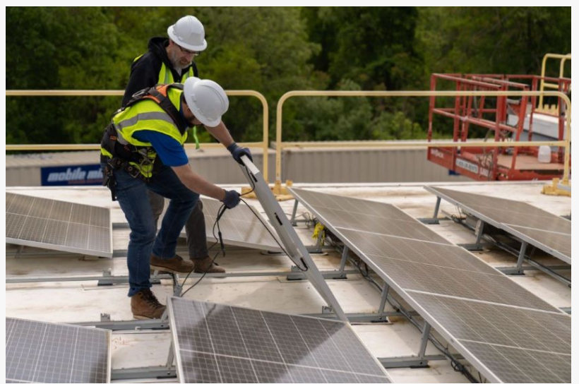
Gridwealth Installs Solar Panel at Ten Mile River Lofts Apartments, 1110 E. Central, Pawtucket, R.I.
