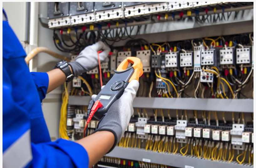
Residential Generator Installation
