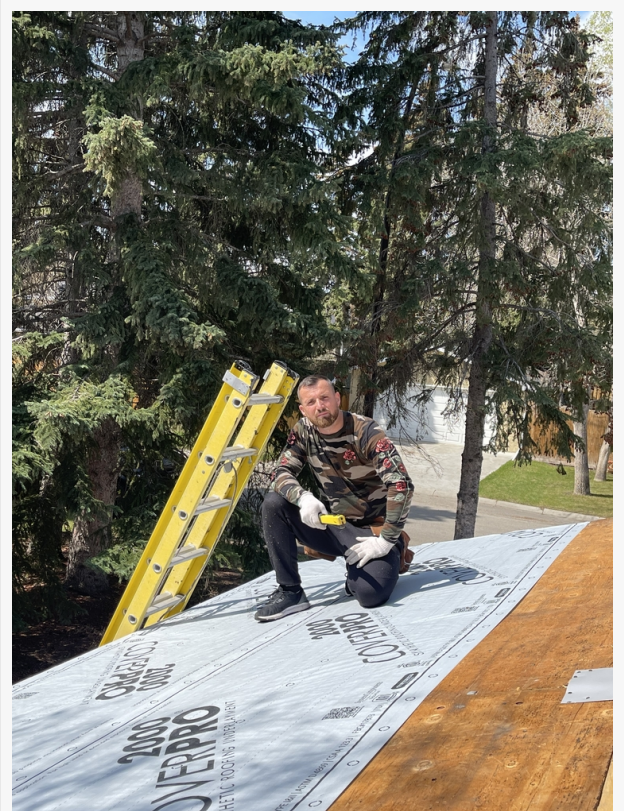
The owner of Calgary Roof Repair Ltd on a roof, Pashk Vukaj.
