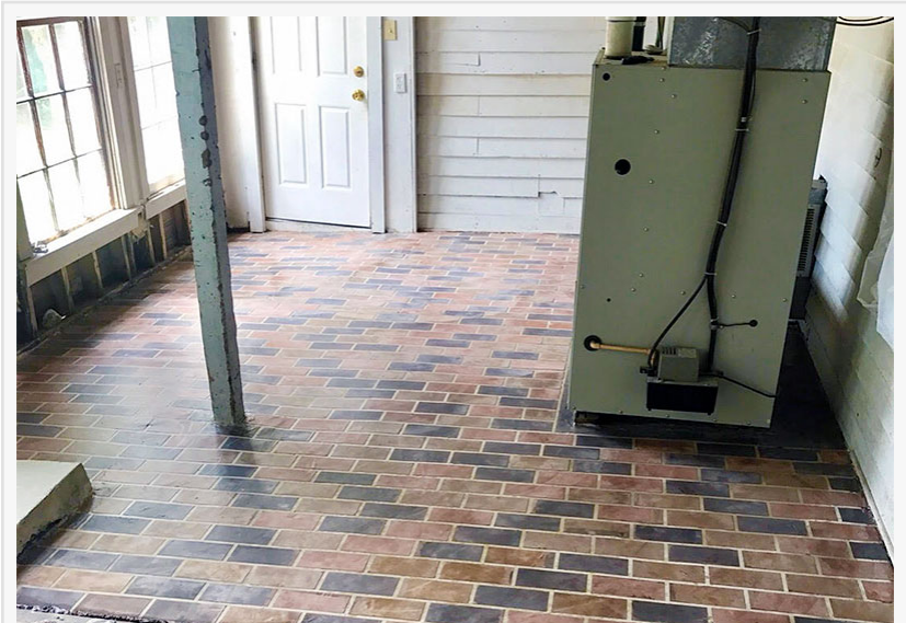
This brick pattern epoxy floor was Dylan and Jake's first paying project.
