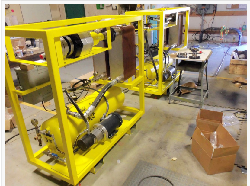
IT10 ORC Turbine Generator which utilizes waste heat for power
