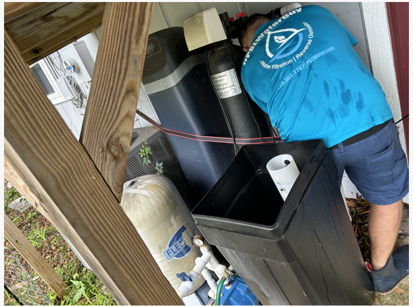
triple system install
