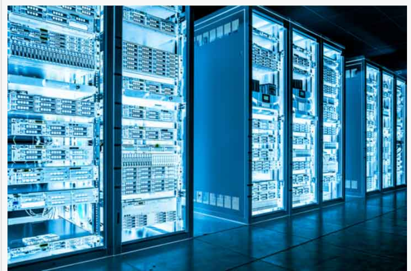
Data Center Power Market
