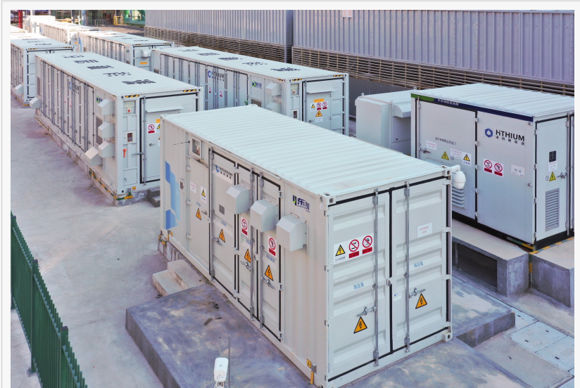
Hithium BESS containers at a 2022 C&I project
