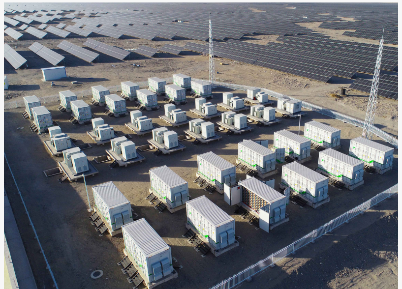
Hithium BESS at 80 MWh solar project
