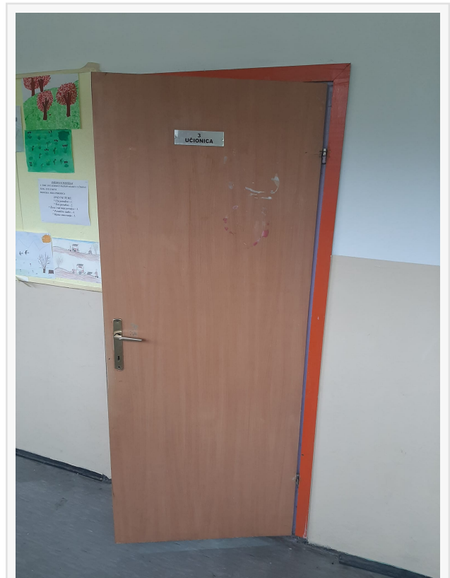
One of five brand-new doors installed by Altenew at this elementary school in Bosnia.
