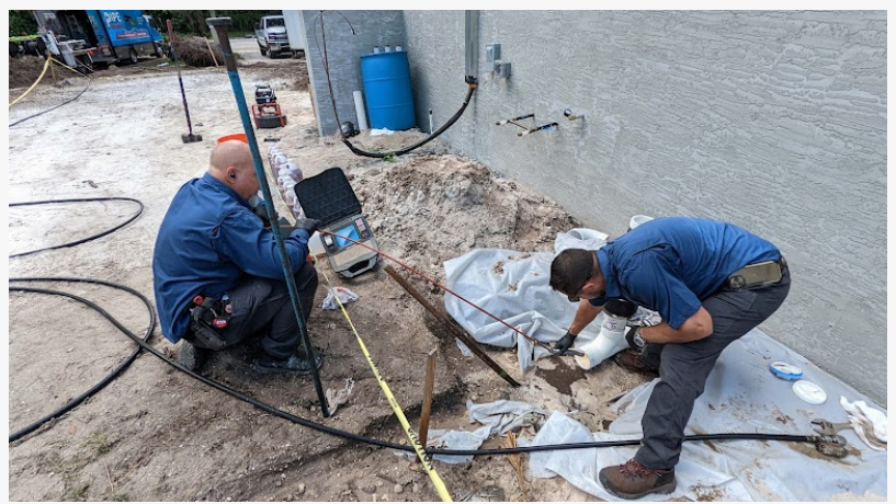
Pipe Surgeons camera inspection services
