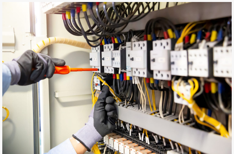
Professional Electrician Services Port St. Lucie and Vero Beach
