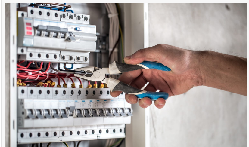
Residential Electrician Services
