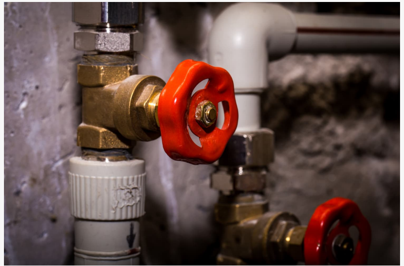
Professional Plumbing Services
