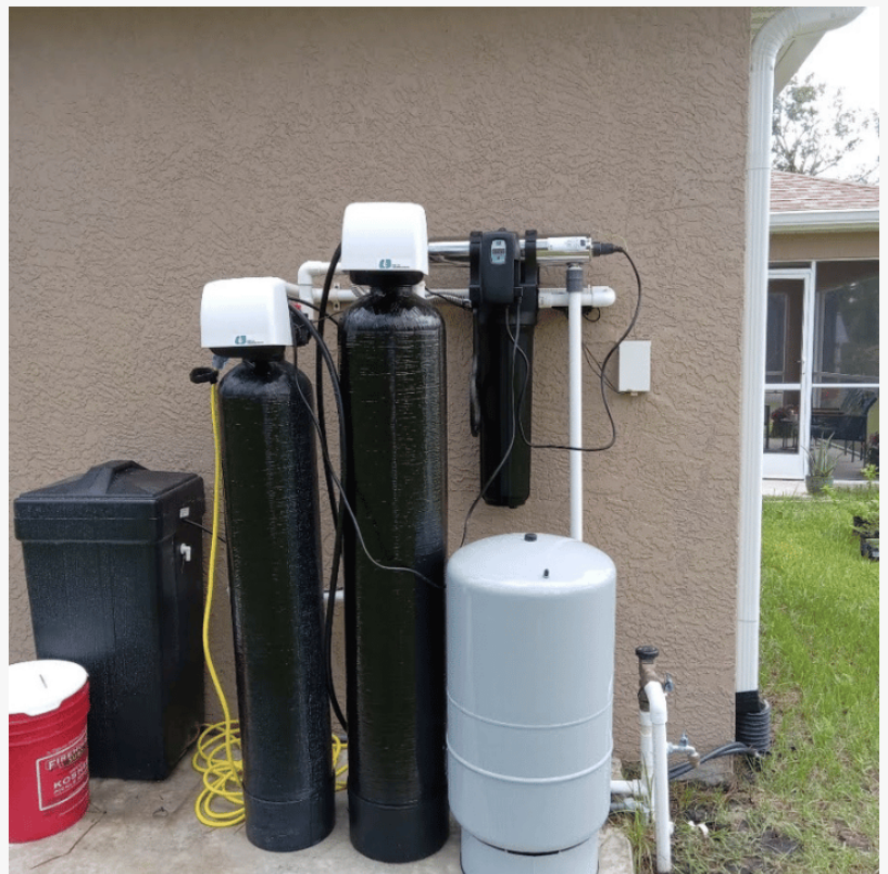
Water Filtration Systems
