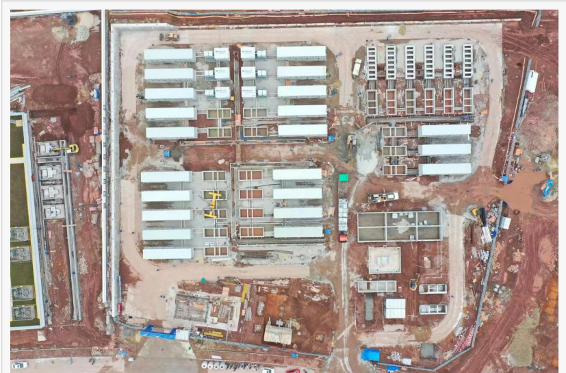
Construction of the 140 MWh CSG plant using Hithium battery systems was completed in four months
