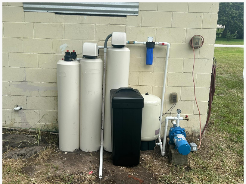
Water Softener System Installation in Port St. Lucie
