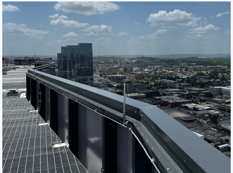
ONE 22 ONE Tower roof with a lightning protection system installed and inspected. Located in Nashville, TN.
