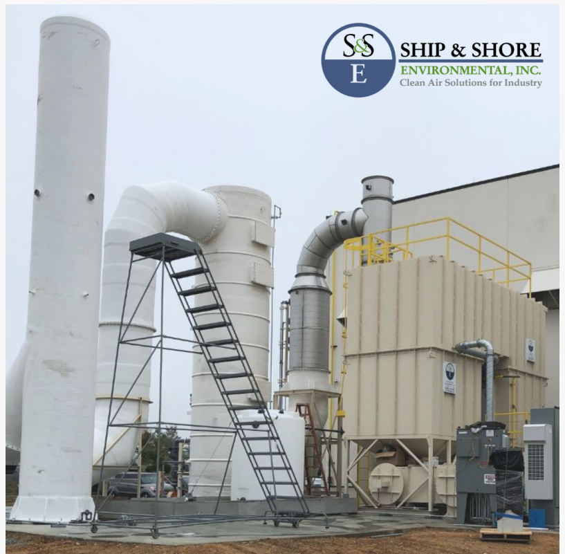
State-of-the-art Ship & Shore Environmental Regenerative Thermal Oxidizer and Scrubber System
