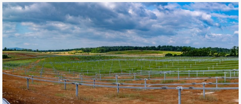
Nevados' All-Terrain Tracker in use on the new 170 MW solar farm.
