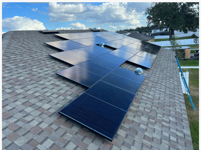
Evergreen Solar Panels on Roof
