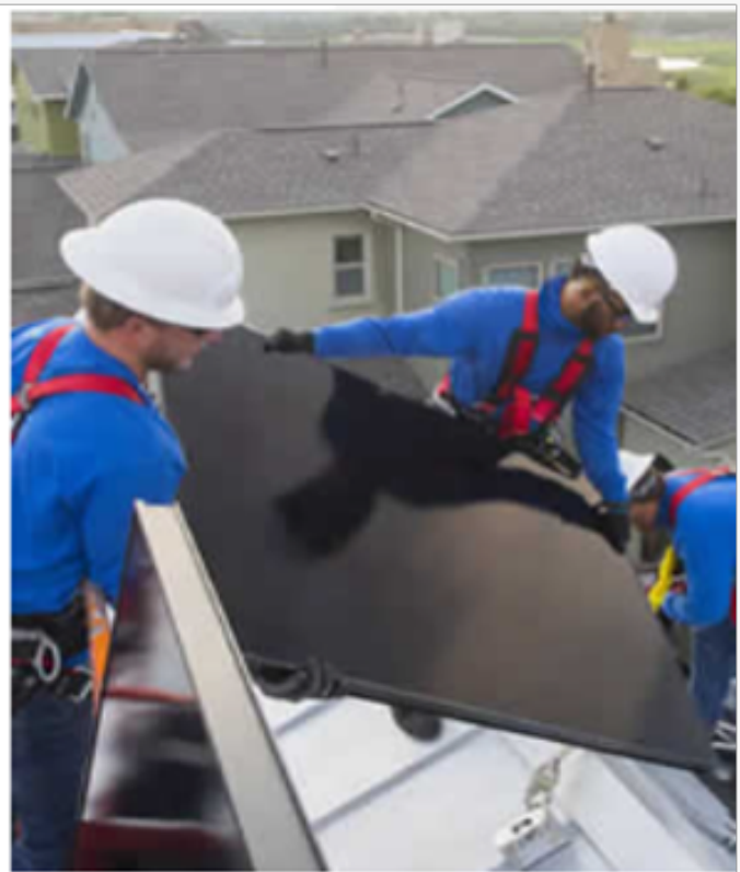
Evergreen Solar Installation
